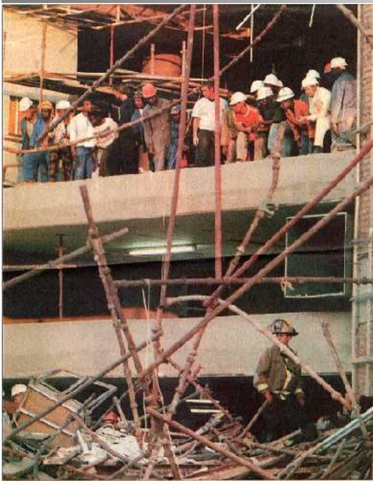
Sombre ... workers survey the scene yesterday at the Investec building where they say heavy marble tiles caused an overload.
