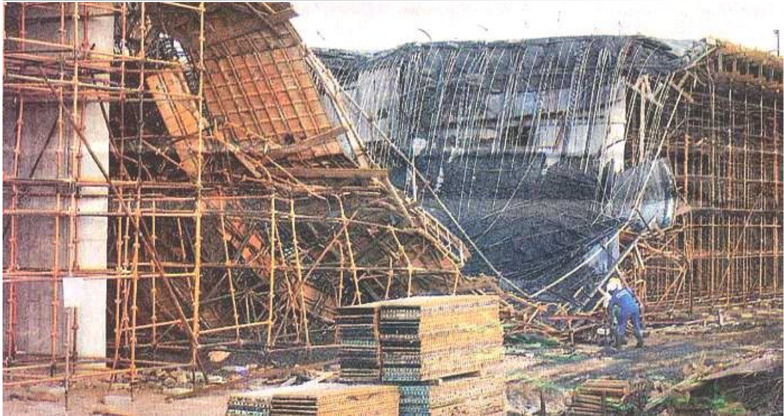
Coega Bridge collapse, Port Elizabeth, November, 2003 (Markman, 2003)
