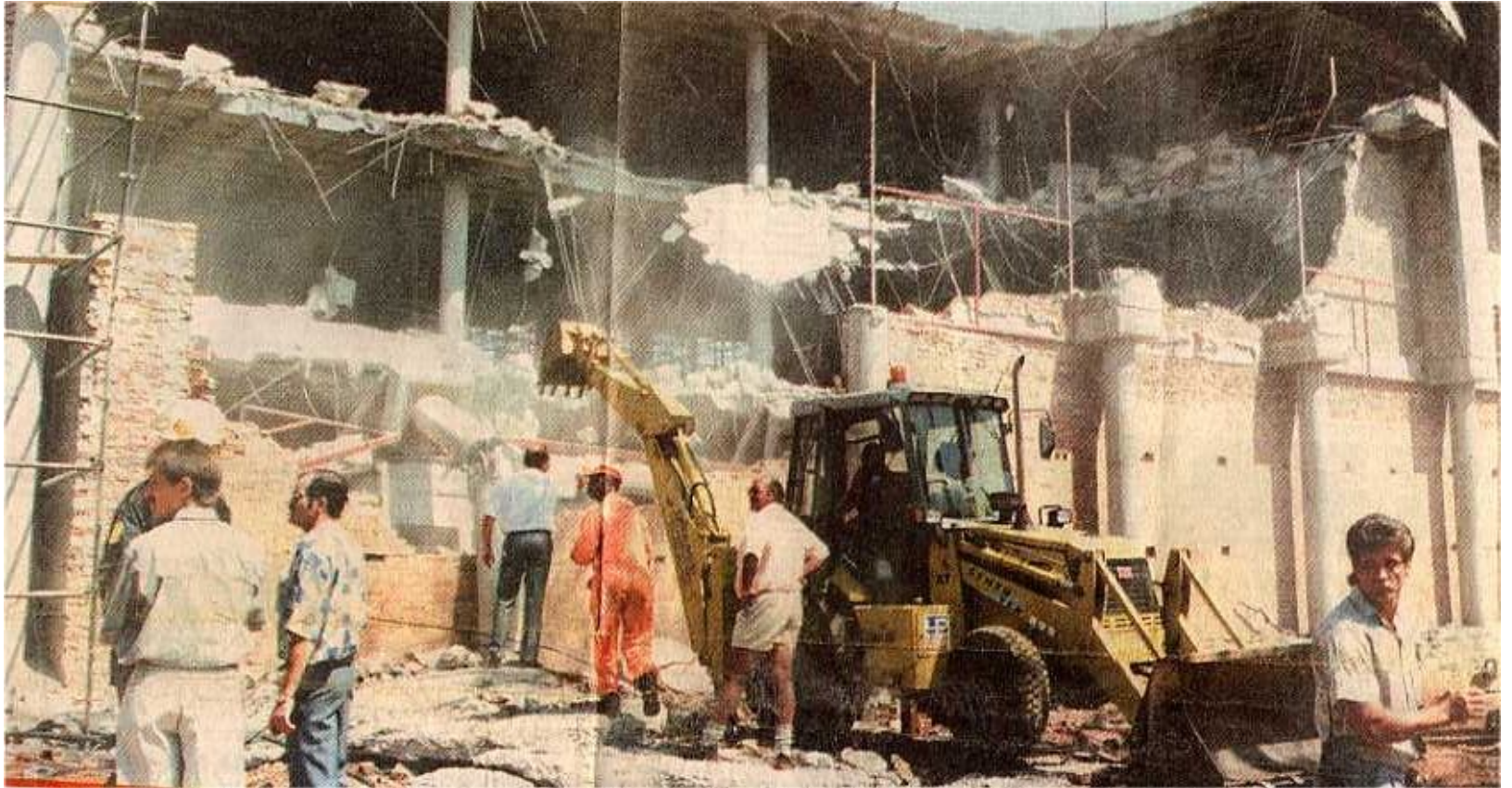
Pretoria North Shopping Centre slab collapse, October, 1996 (Davis, 1996)
