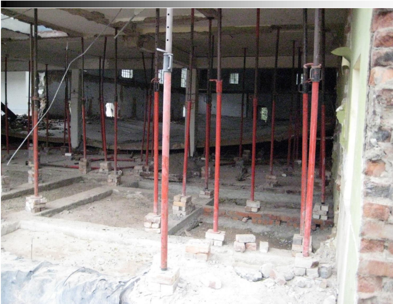
Stellenbosch Collapse (Anonymous, June 2008)
