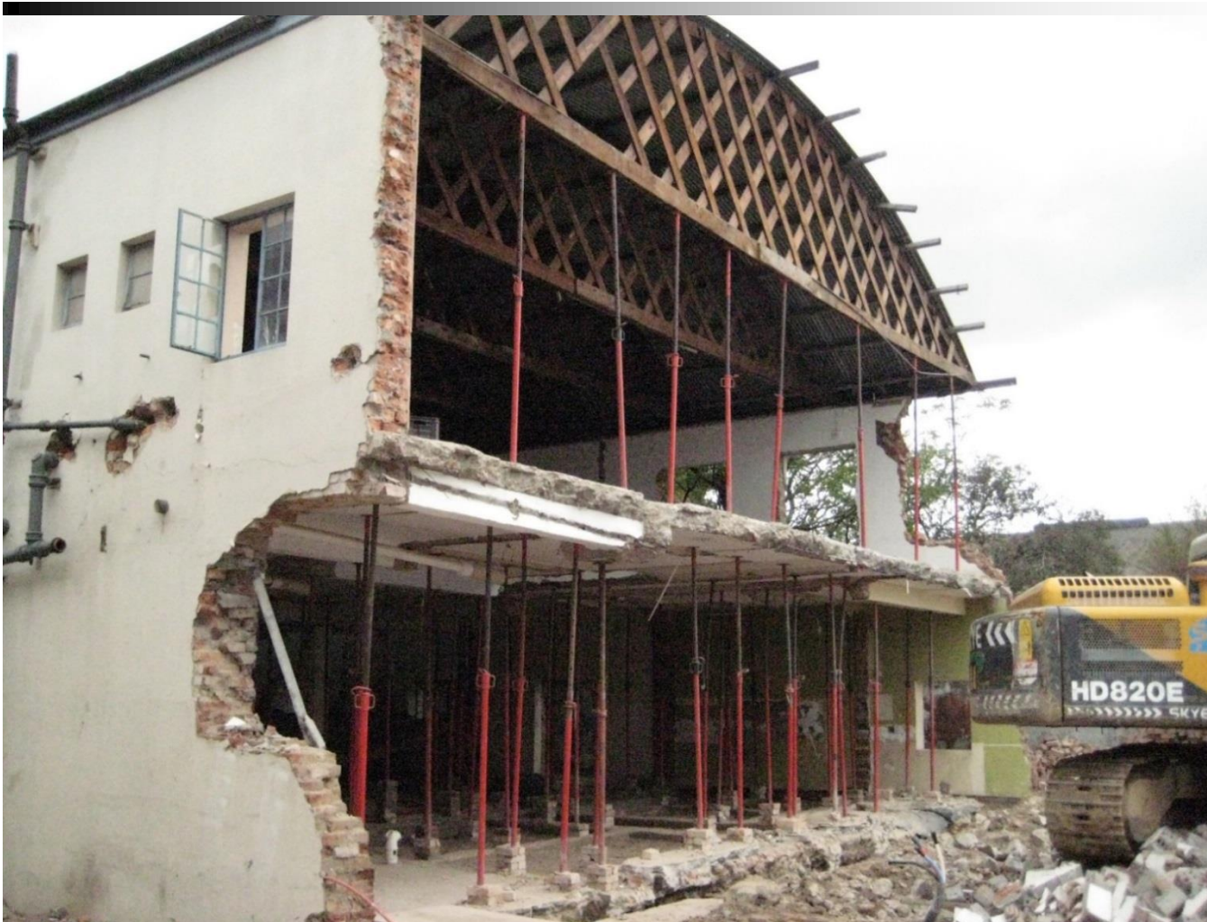
Stellenbosch Collapse (Anonymous, June 2008)
