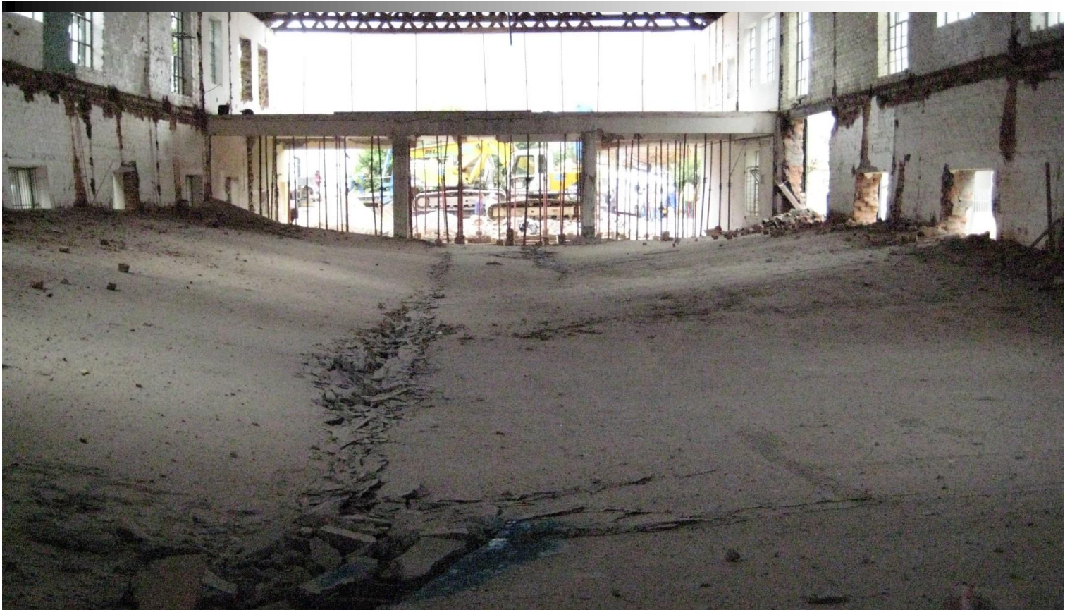
Stellenbosch Collapse (Anonymous, June 2008)
