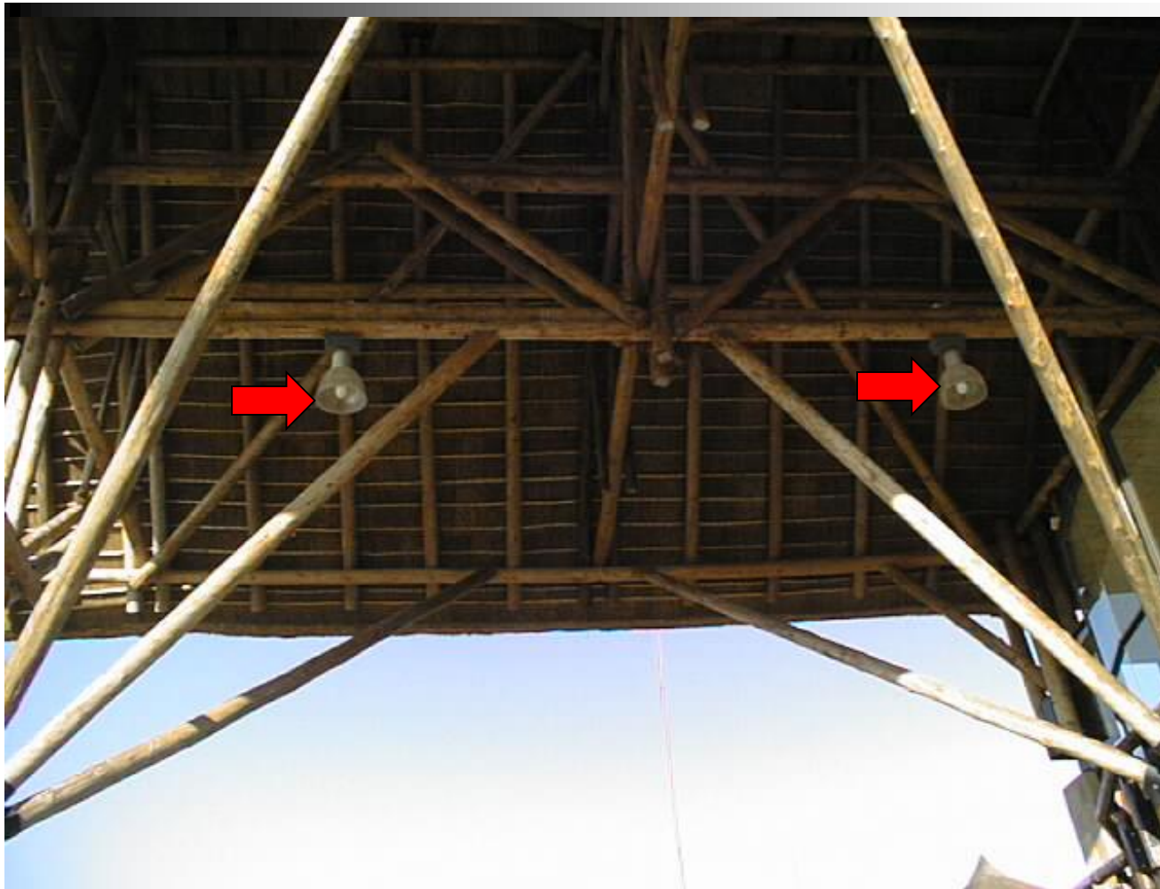
Light fittings, Porte Cochere, Nelspruit Airport (Smallwood, 2004)
