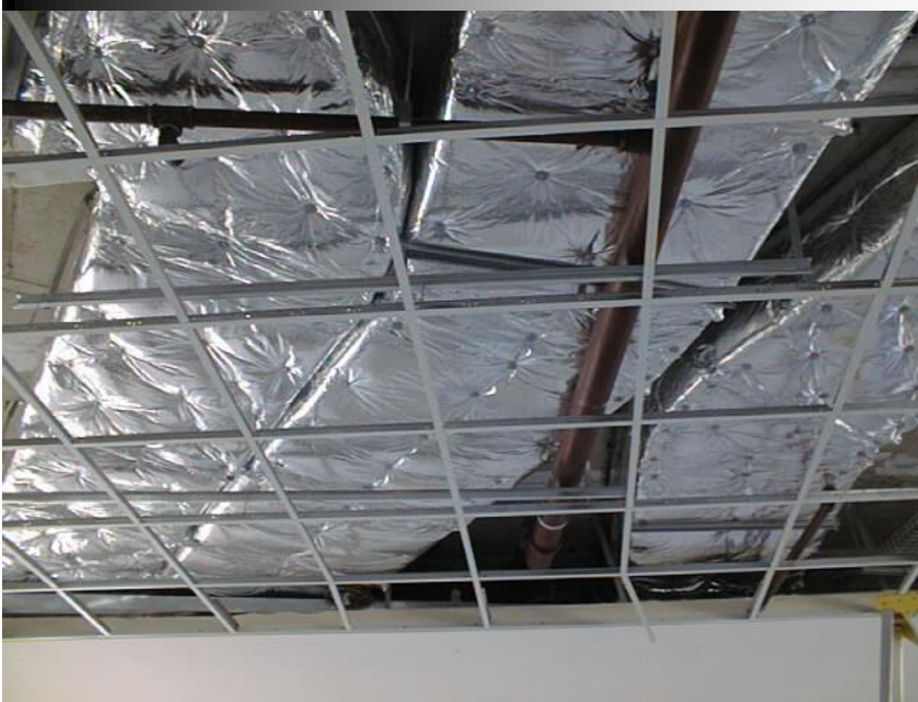
Congested ceiling space, Cape Town (Smallwood, 2004)
