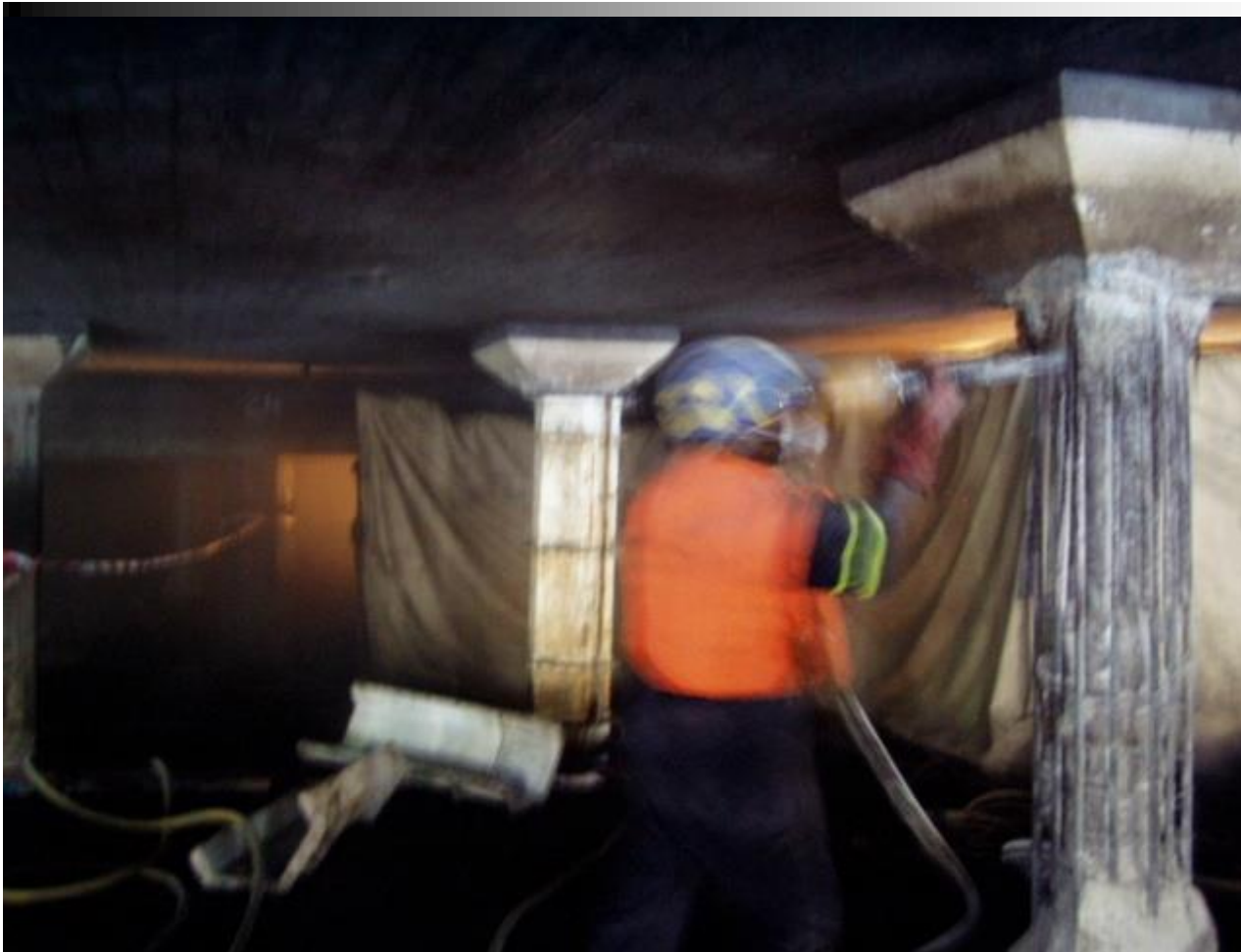
Exposing of corroded steel to piers beneath Dar Es Salaam Quay (Deacon, 2005)
