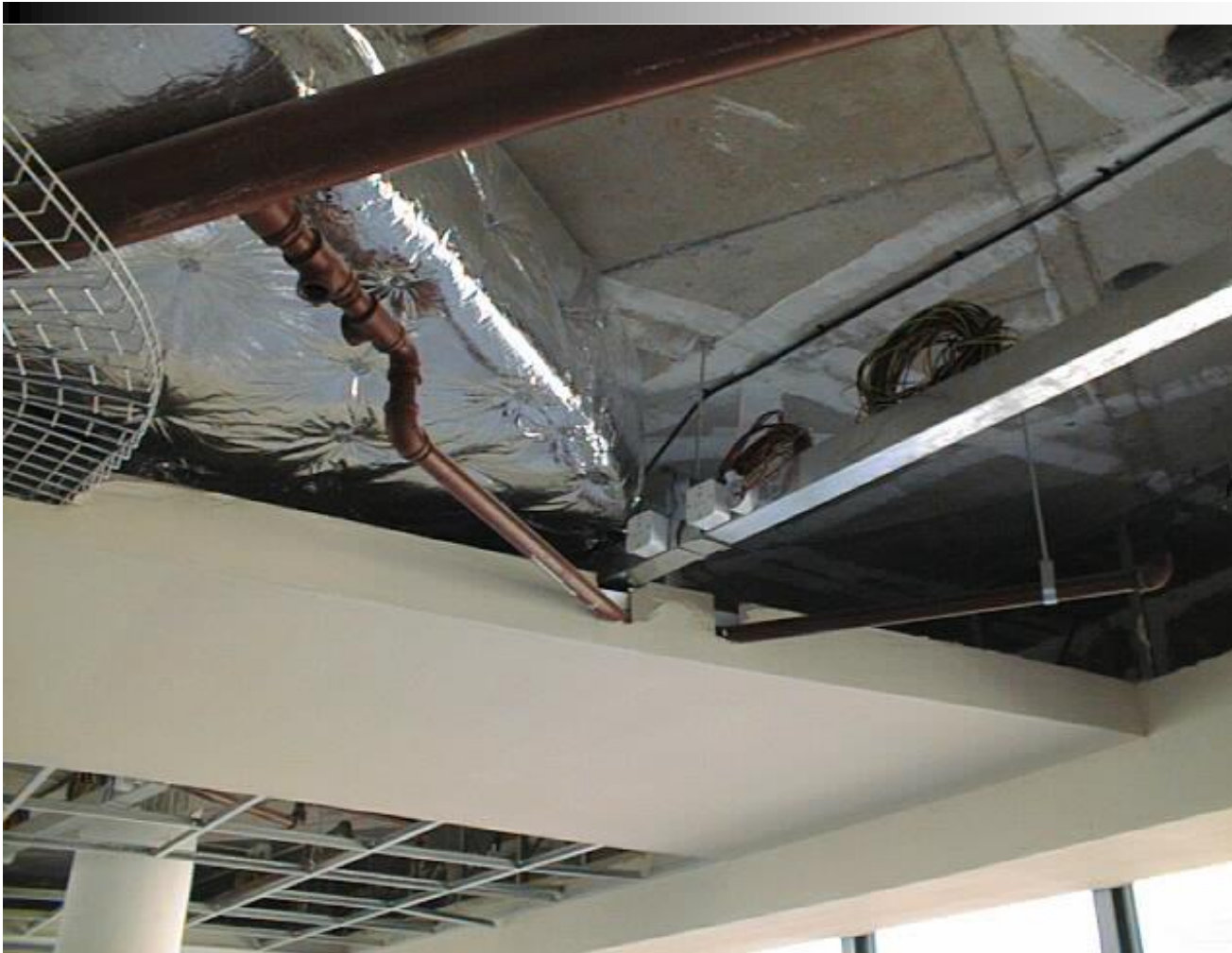
Congested ceiling space, Cape Town (Smallwood, 2004)
