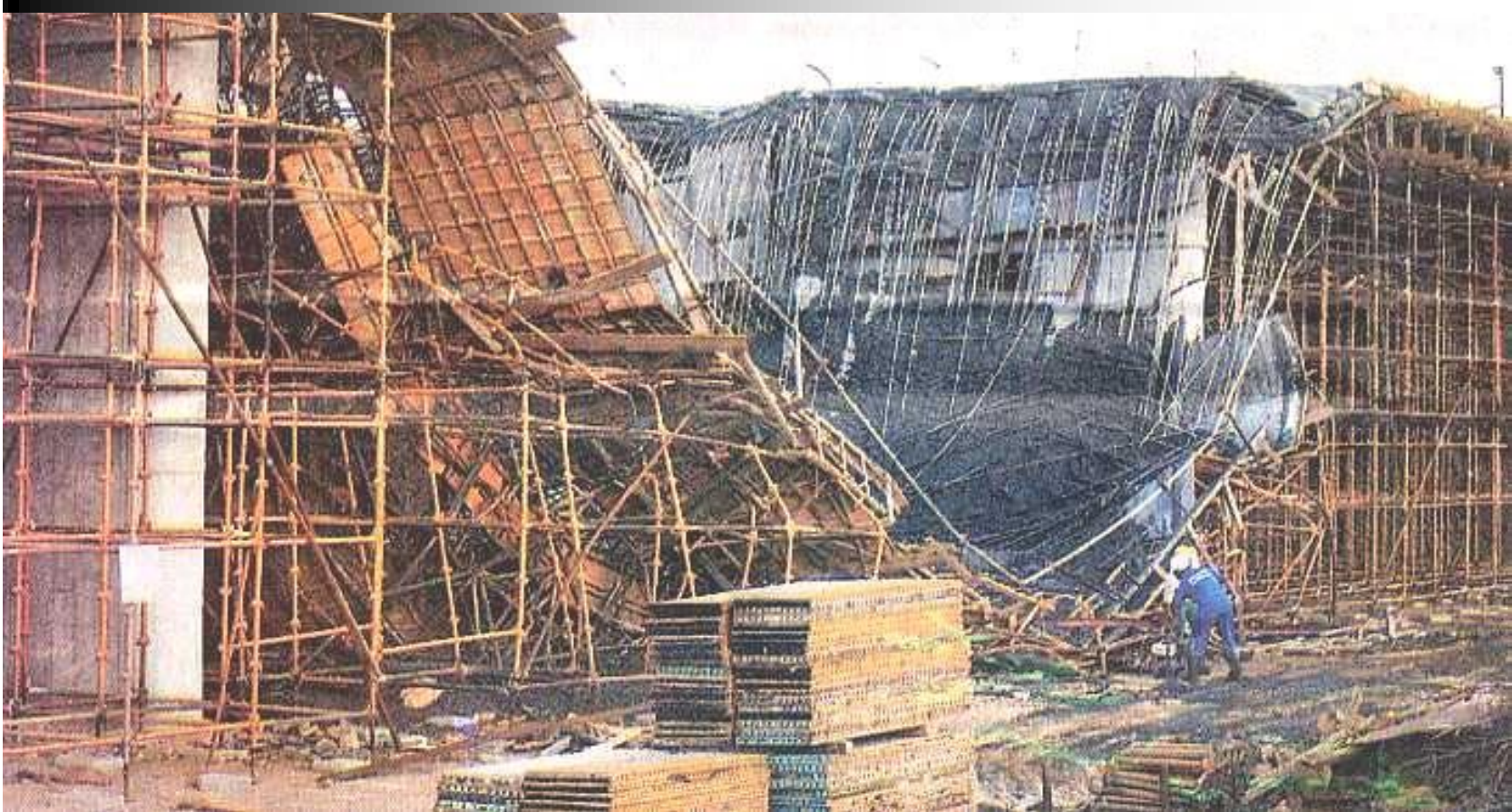
Coega Bridge collapse, Port Elizabeth, November, 2003 (Markman, 2003)
