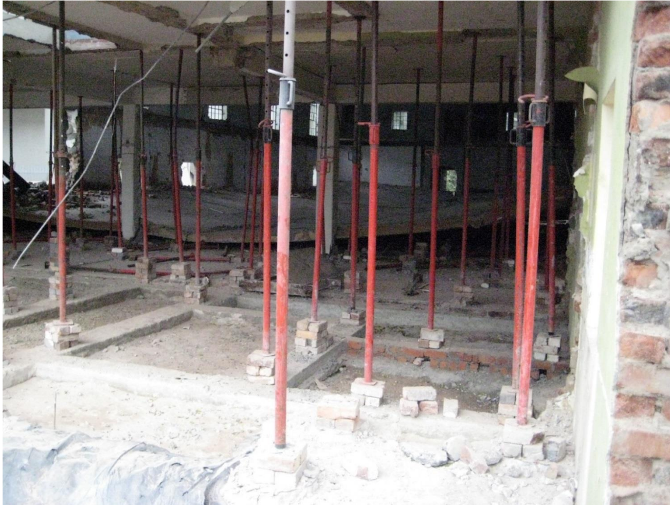
Stellenbosch Collapse (Anonymous, June 2008)
