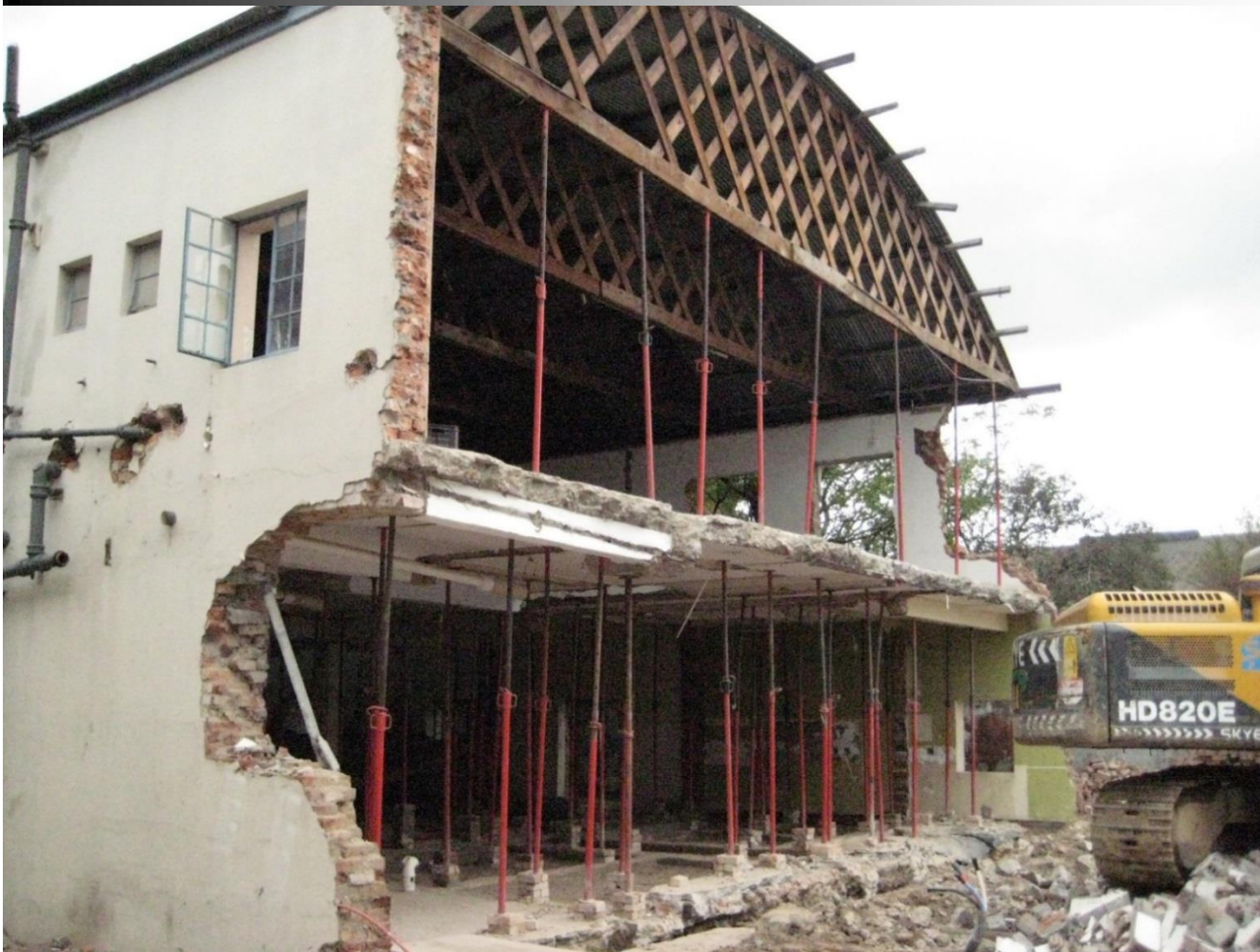
Stellenbosch Collapse (Anonymous, June 2008)
