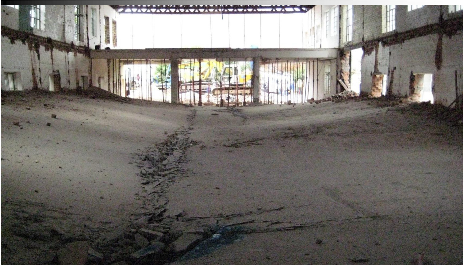
Stellenbosch Collapse (Anonymous, June 2008)
