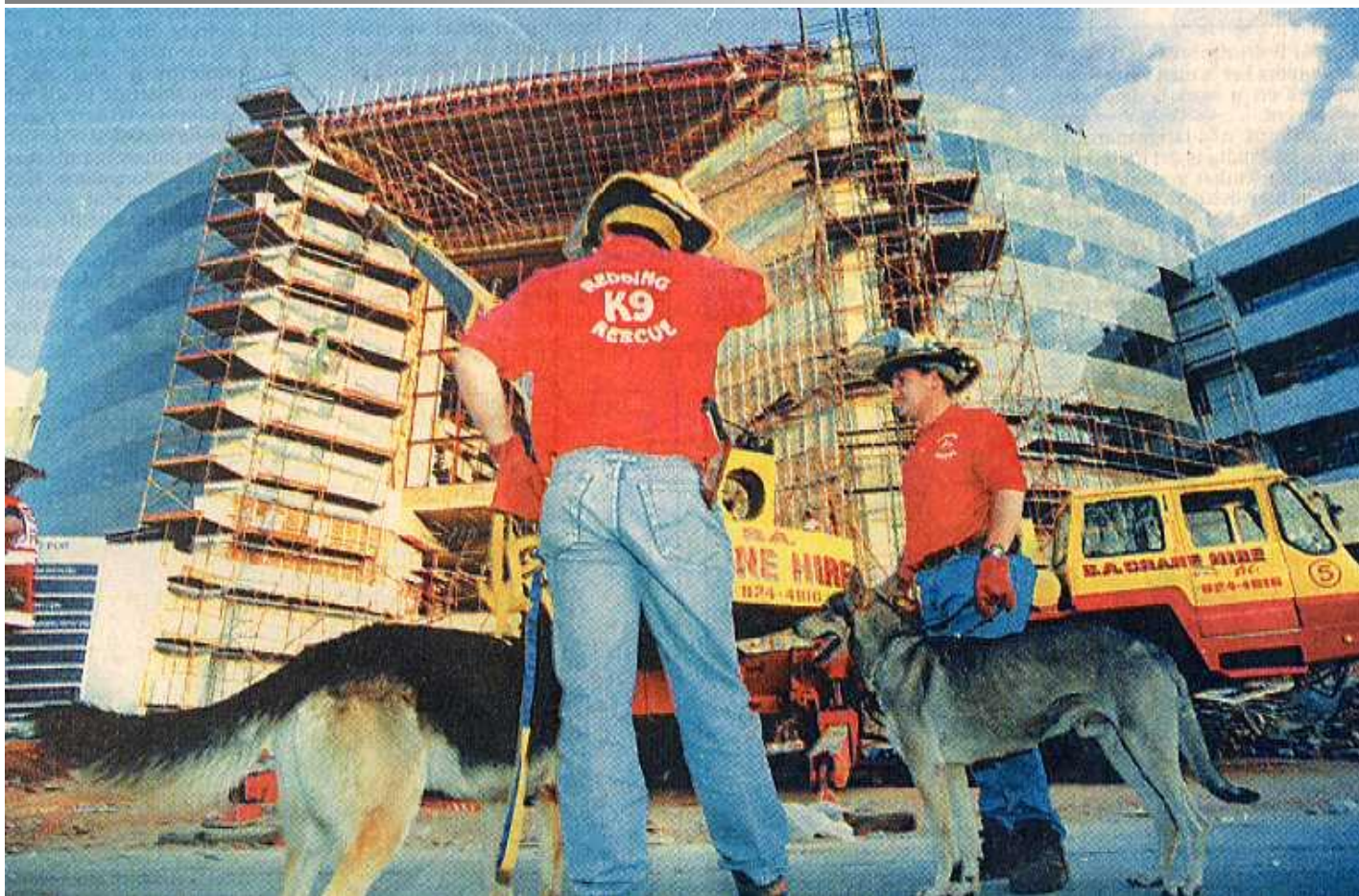
Investec Office Complex scaffolding collapse, Sandton, August, 1997 (Prinsloo, 1997)
