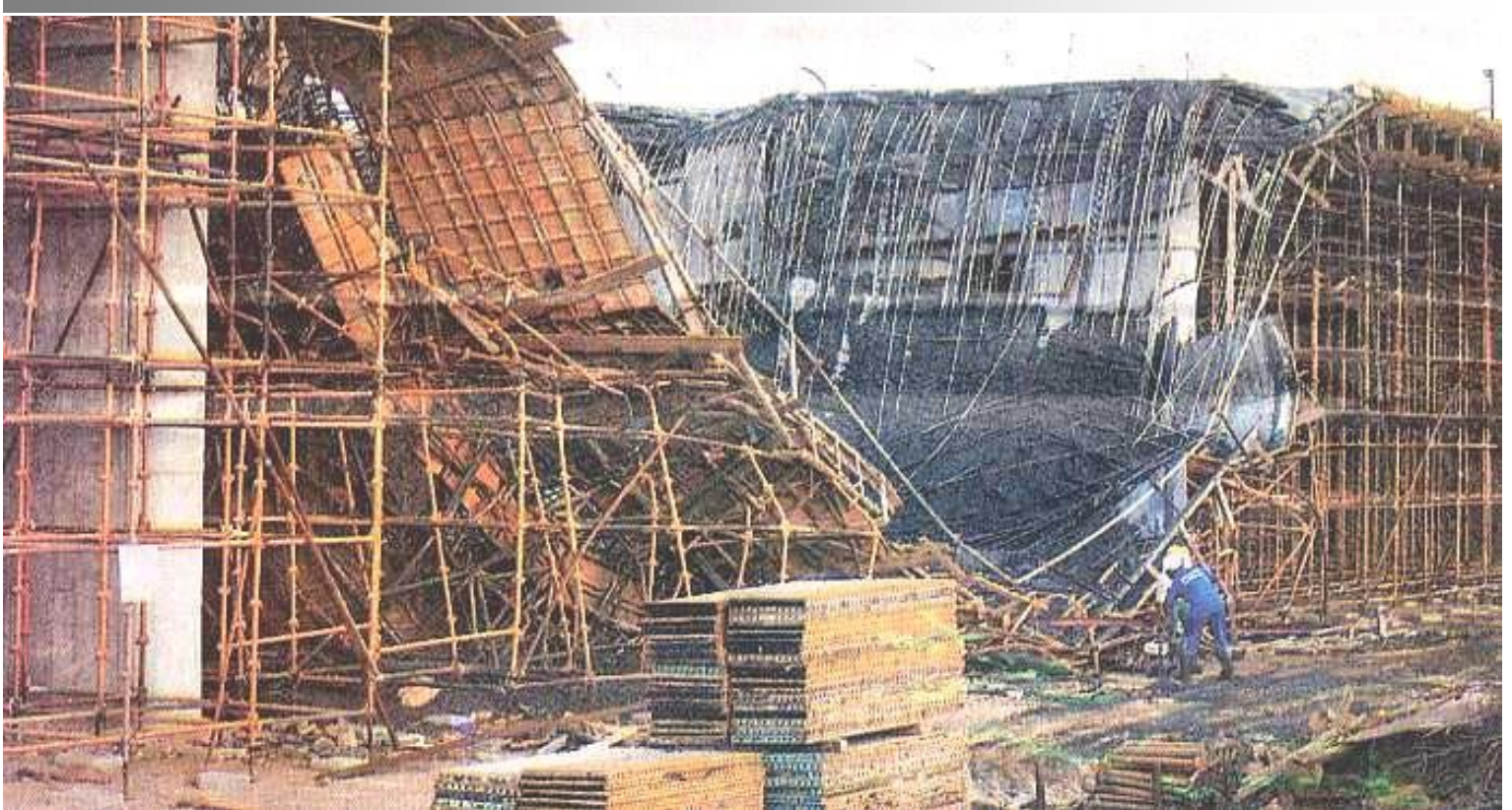
Coega Bridge collapse, Port Elizabeth, November, 2003 (Markman, 2003)
