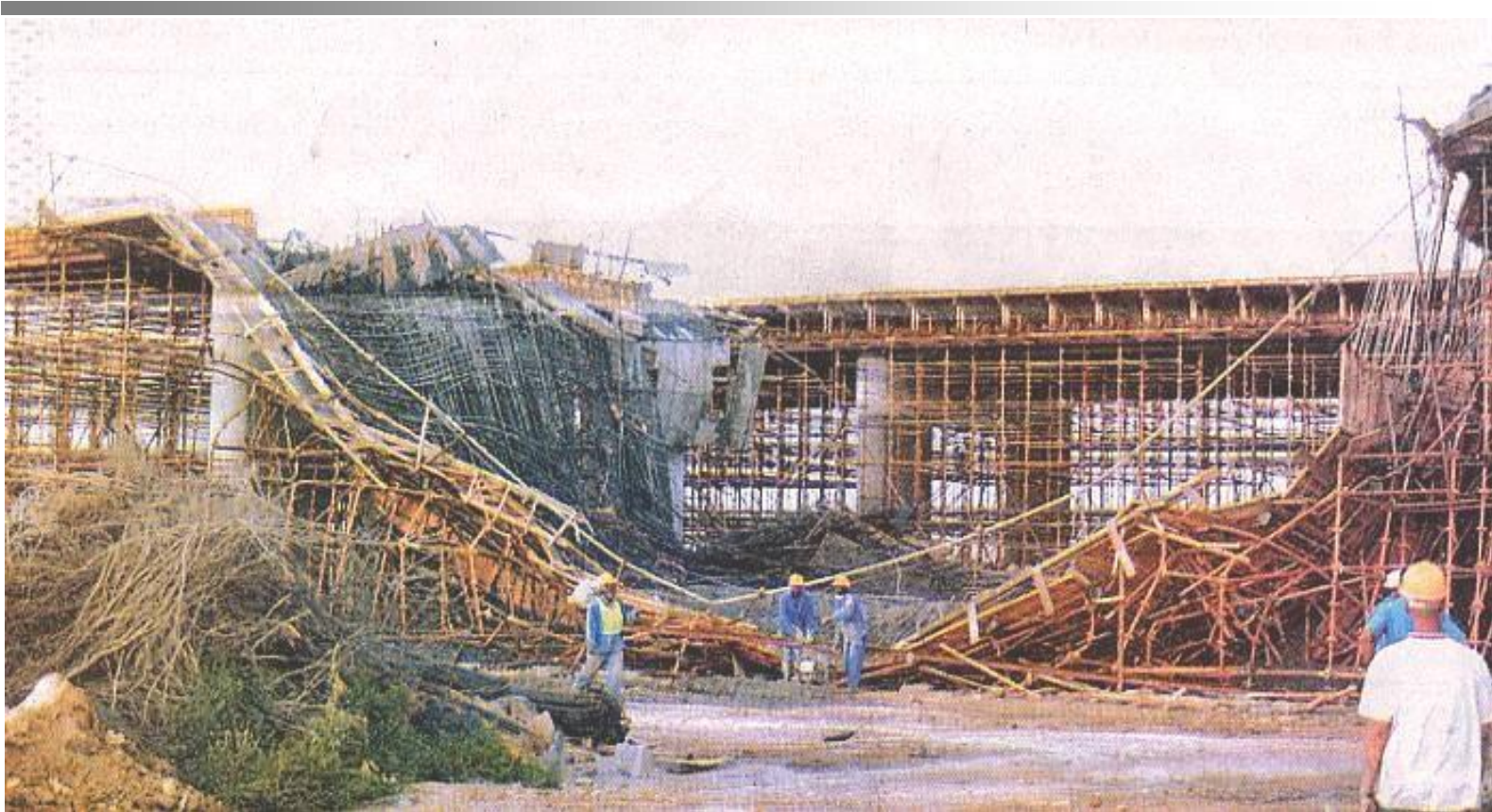
Coega Bridge collapse, Port Elizabeth, November, 2003 (Markman, 2003)
