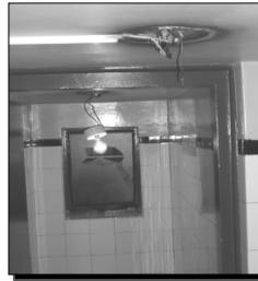
Low hanging toilet lighting
