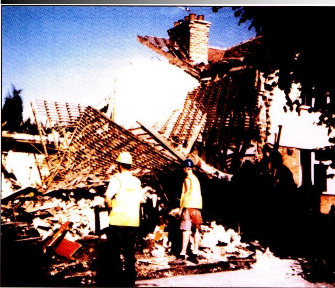
Aftermath of a gas explosion following damage to an underground gas service pipe (HSE, 2000)
