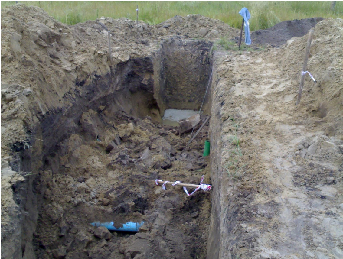
Trench collapse, Umhlathuze Municipality, 2007 (Umhlathuze Municipality Excavation H&S Seminar Delegate, 2007)
