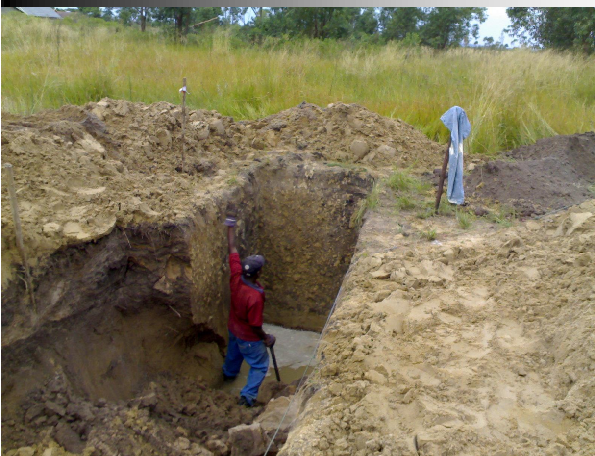
Trench collapse, Umhlathuze Municipality, 2007 (Umhlathuze Municipality Excavation H&S Seminar Delegate, 2007)
