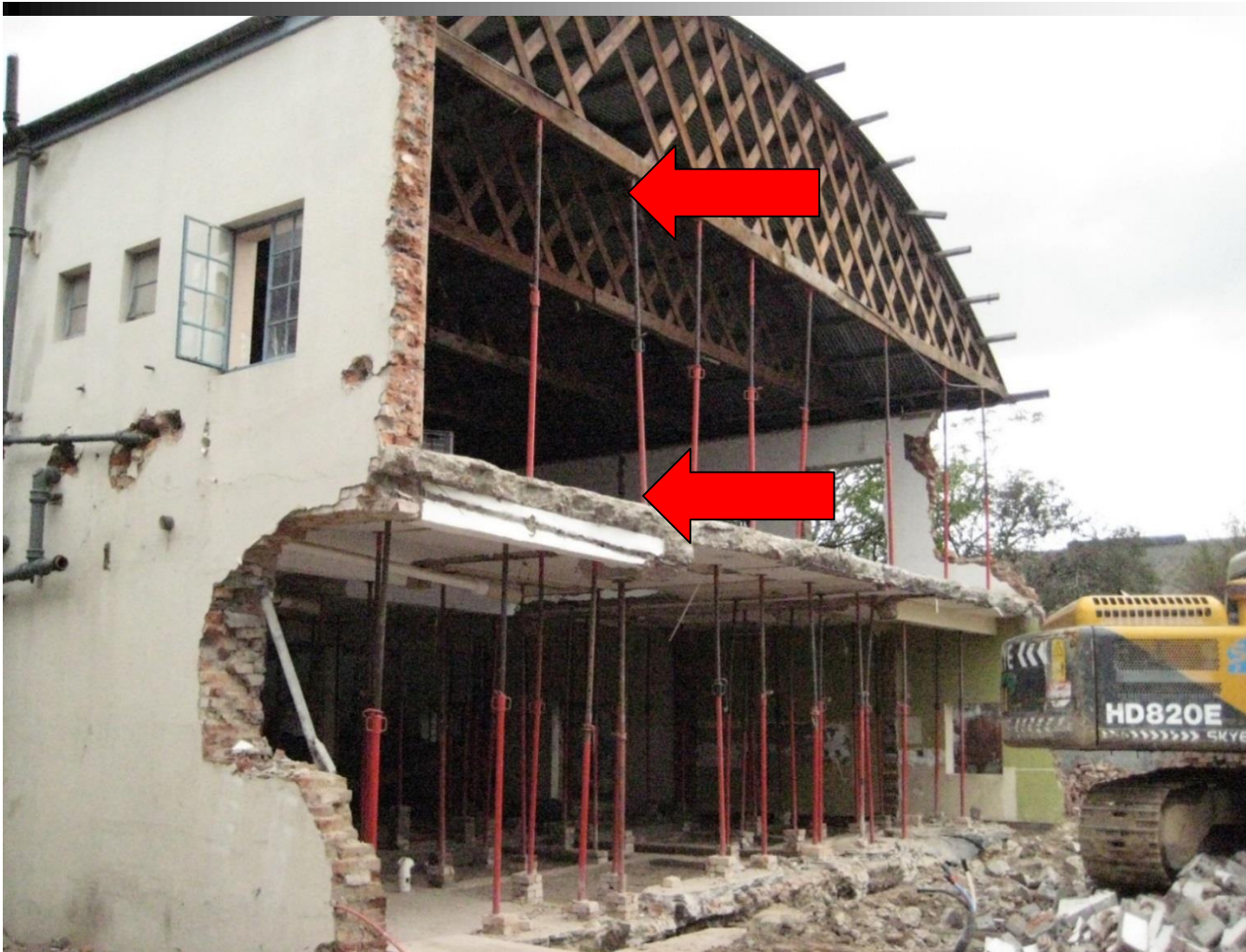
Stellenbosch Collapse (Anonymous, June 2008)
