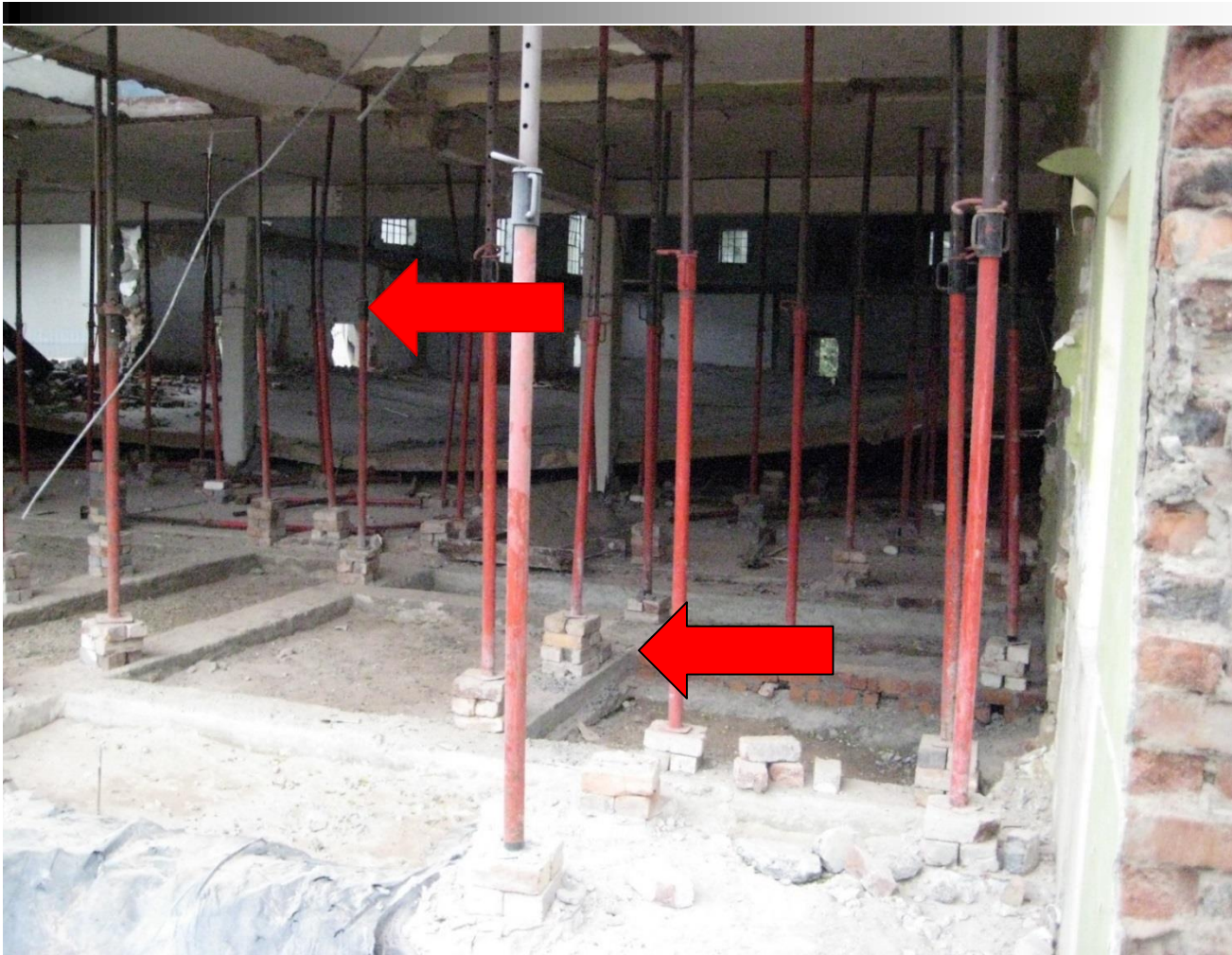
Stellenbosch Collapse (Anonymous, June 2008)
