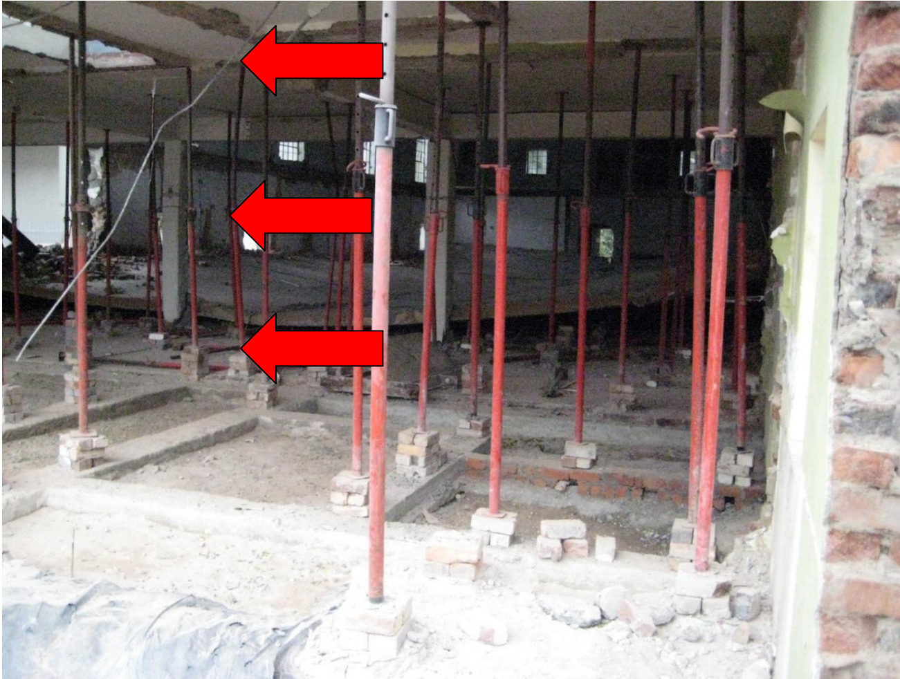
Stellenbosch Collapse (Anonymous, June 2008)
