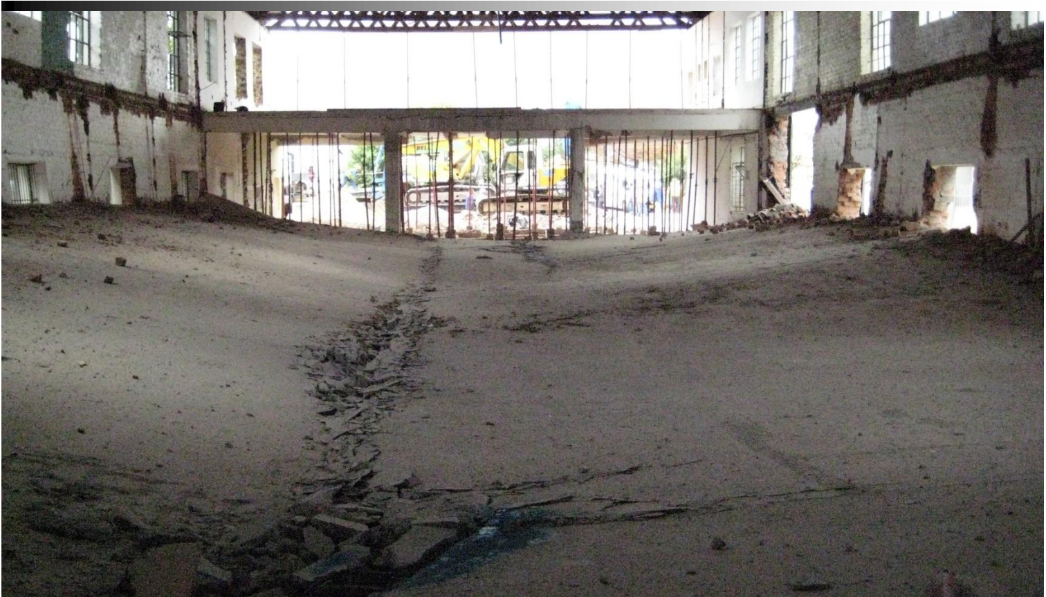
Stellenbosch Collapse (Anonymous, June 2008)
