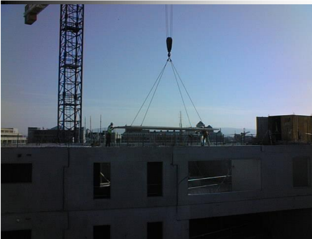
Precast floor panels, Dublin (Smallwood, 2004)
