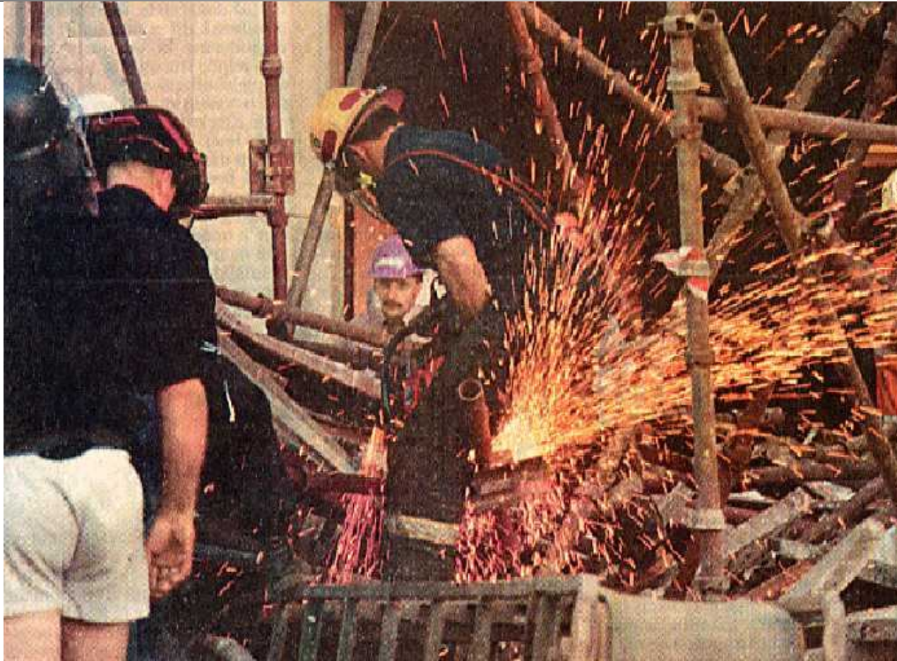
Investec Office Complex scaffolding collapse, Sandton, August, 1997 (Prinsloo, 1997)
